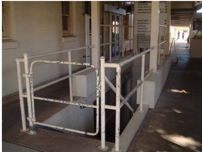
Stairs down to Calorifier room under Admissions and Discharges (12)
