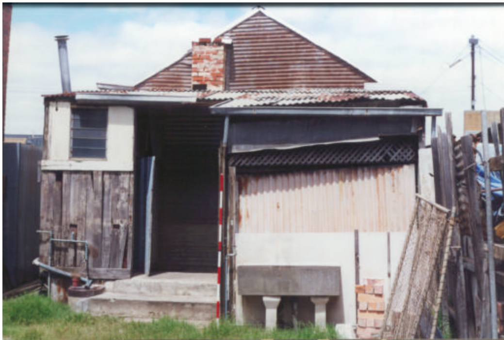
Figure 2: A view of the rear of 15 Quebec Street, Port Adelaide (Photo: Susan Briggs)
